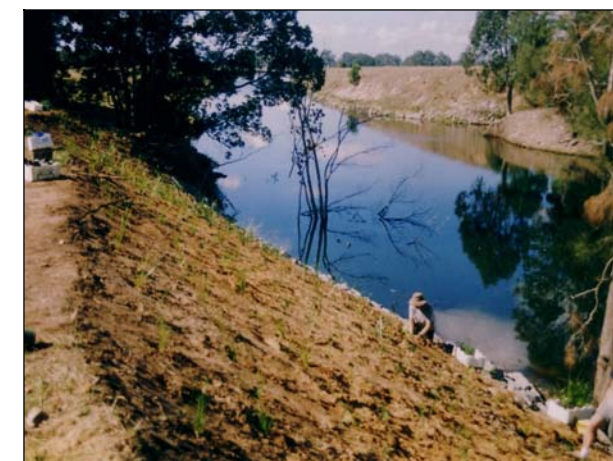
Revegetation of streambank to prevent erosion. Here the streambank was re-battered after slumping (note the loss of bank, and dead trees in the water (photo J. Green)
